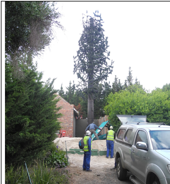
Figure 1 - Dalham Road "tree" Mast
